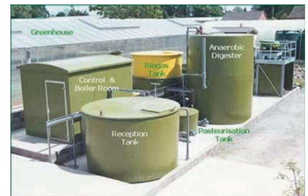
Figure 61: Anaerobic Digestion Equipment
